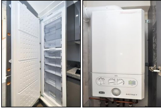
Full Height Freezer, 'A' rated boiler
